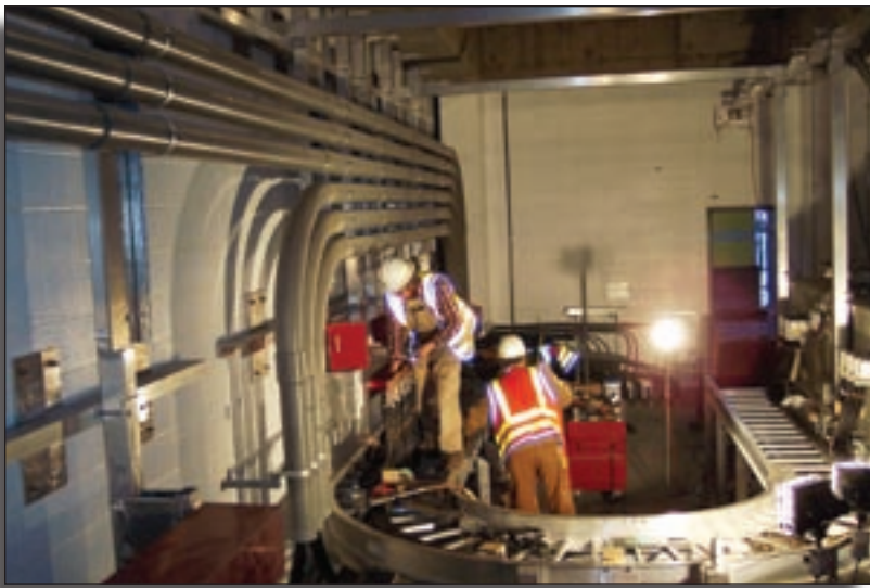
Theresa Hansen (left) and Bill Welborn were among the Tacoma Power electricians whose experience, skills and strength were required to install electrical service to the new Tacoma convention center.
